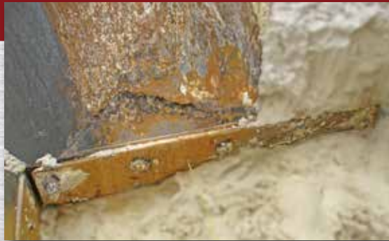
Standard steel liners = Downtime (and lots of it!), outages, material loss, maintenance costs, and quality issues.
